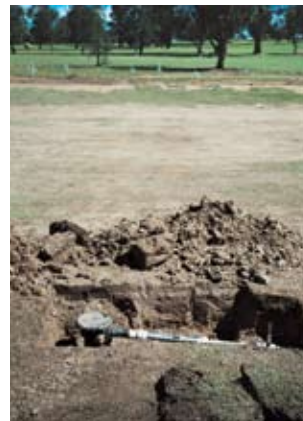
CF40 at sprinkler head
