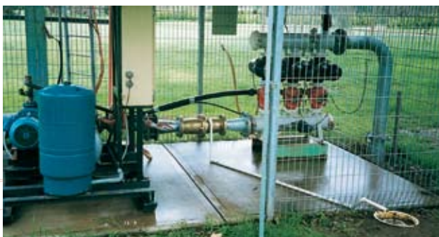
100mm Care-Free Conditioner installed into a 150mm line at the golf course. Flowrate: 2700 lit/min Headloss: 41kPa – no orifice.
