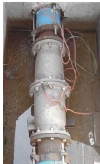
150mm Care-Free Conditioner turns over entire lake every 36 hours. Flowrate 6,000 lit/min.
